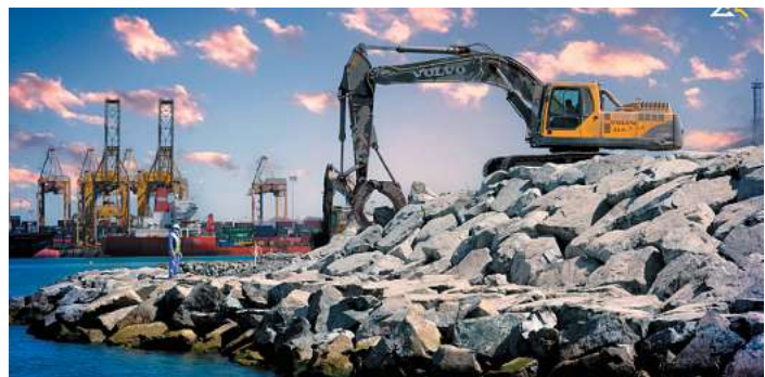
Gulf Rock performs rock placement to protect land embankments and build marine structures.
